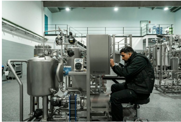
Scheduled maintenance keeps premises and equipment in good working order.
