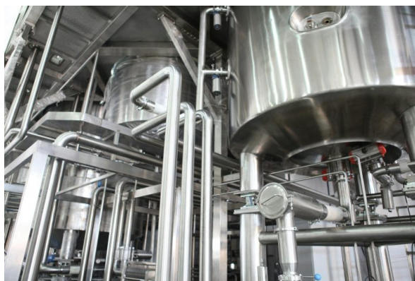
Stainless steel vessels and pipework in a food processing facility.
